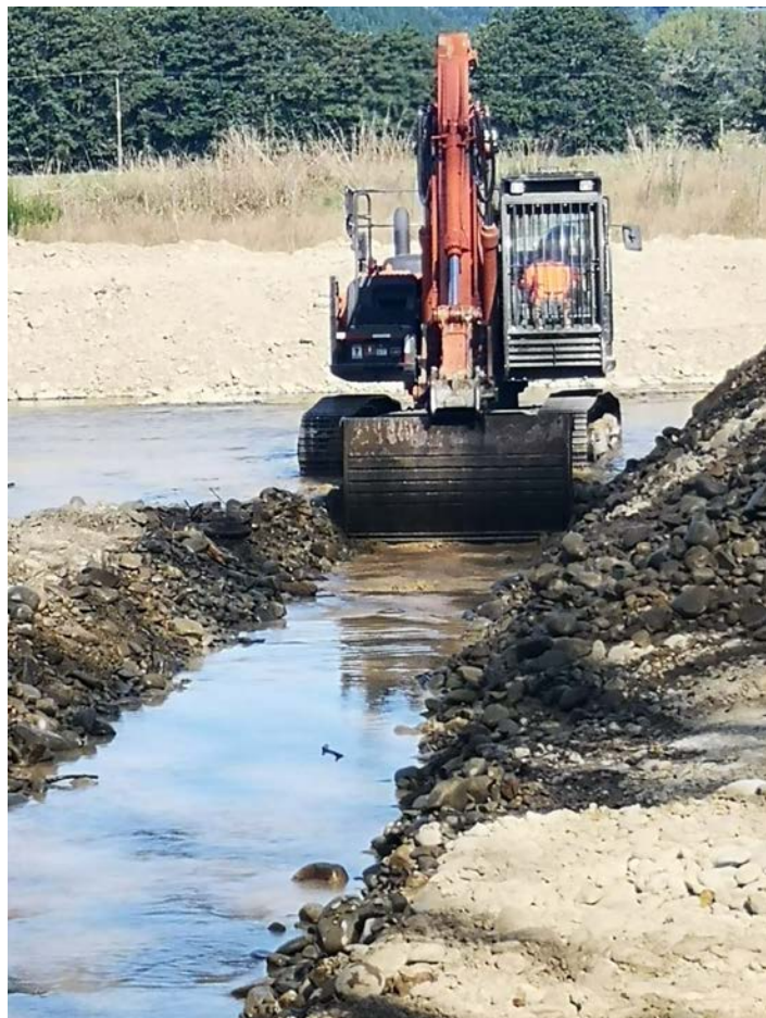
v A trench was dug from the main Motupiko to the stranded fish to encourage the trout to return to the main river.
